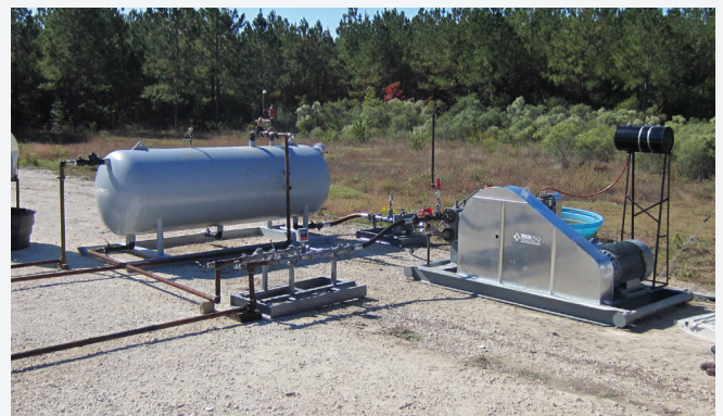
Permanent installation after production testing with a natural gas unit.
